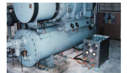
Lubricating oil for the 150 kw screw compressor (SRC-814-C)
