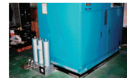
Lubricating oil for the 75 kw screw compressor (SRC-813-C)
